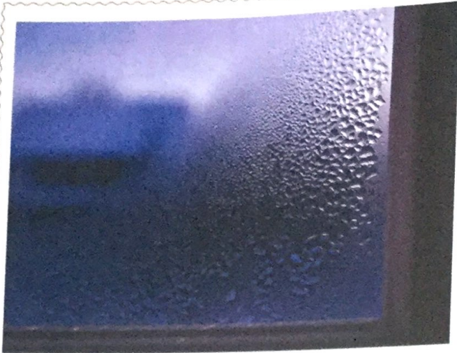
Condensation on a window
